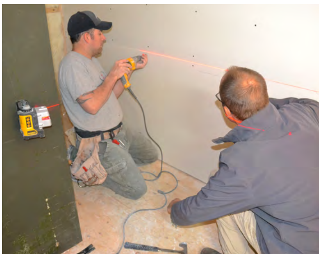
David Beaudriault (left) and Didier Thomas (right) are busy installing drywall sheets.
